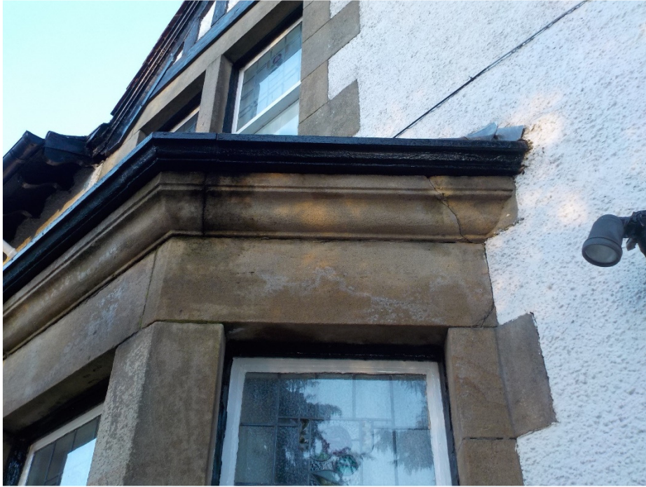
Photograph No.5 – Cracked stone cornice
