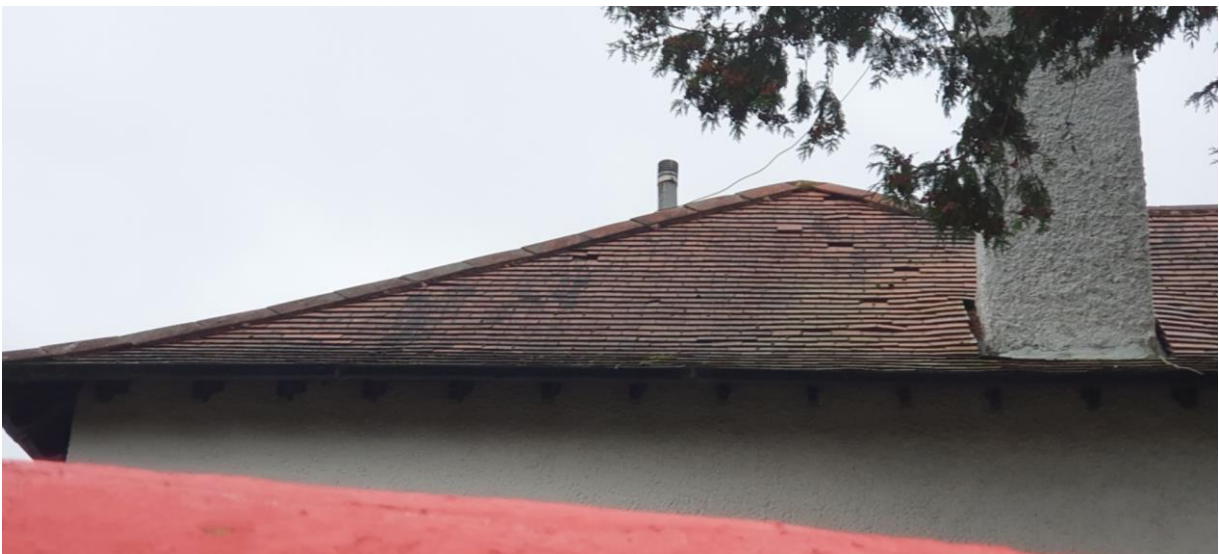
Plate 10. Typical PRF on roof - missing tiles/damage
