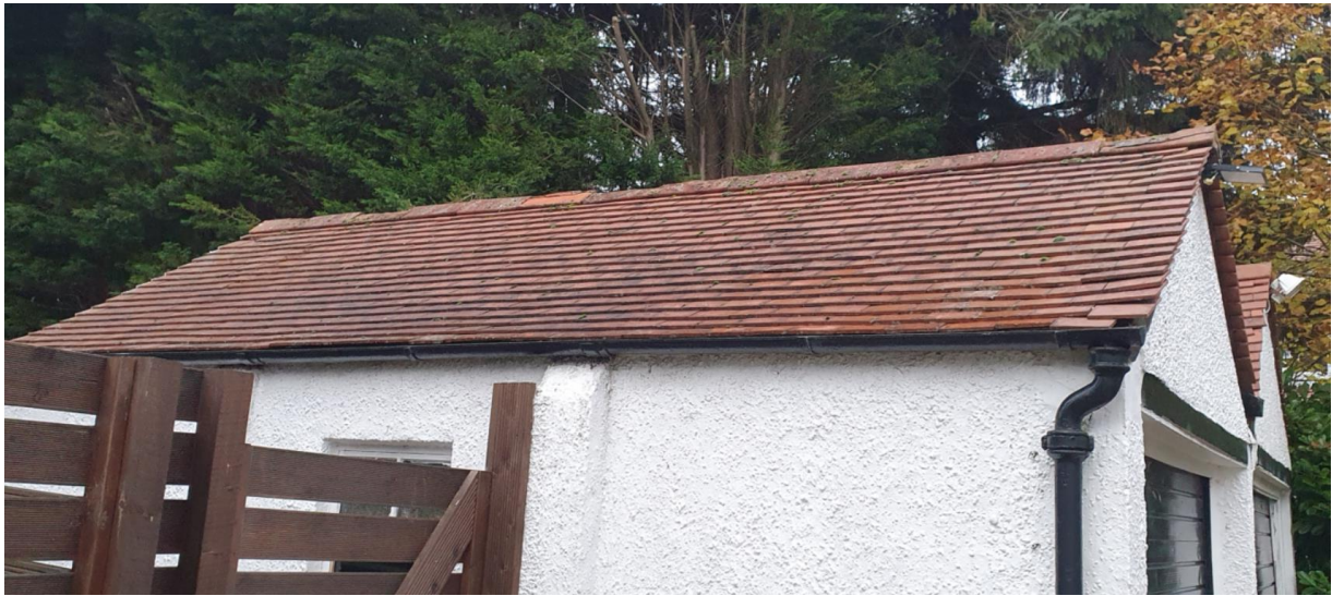
Plate 5. Building B2 showing gaps in roofing (right end)
