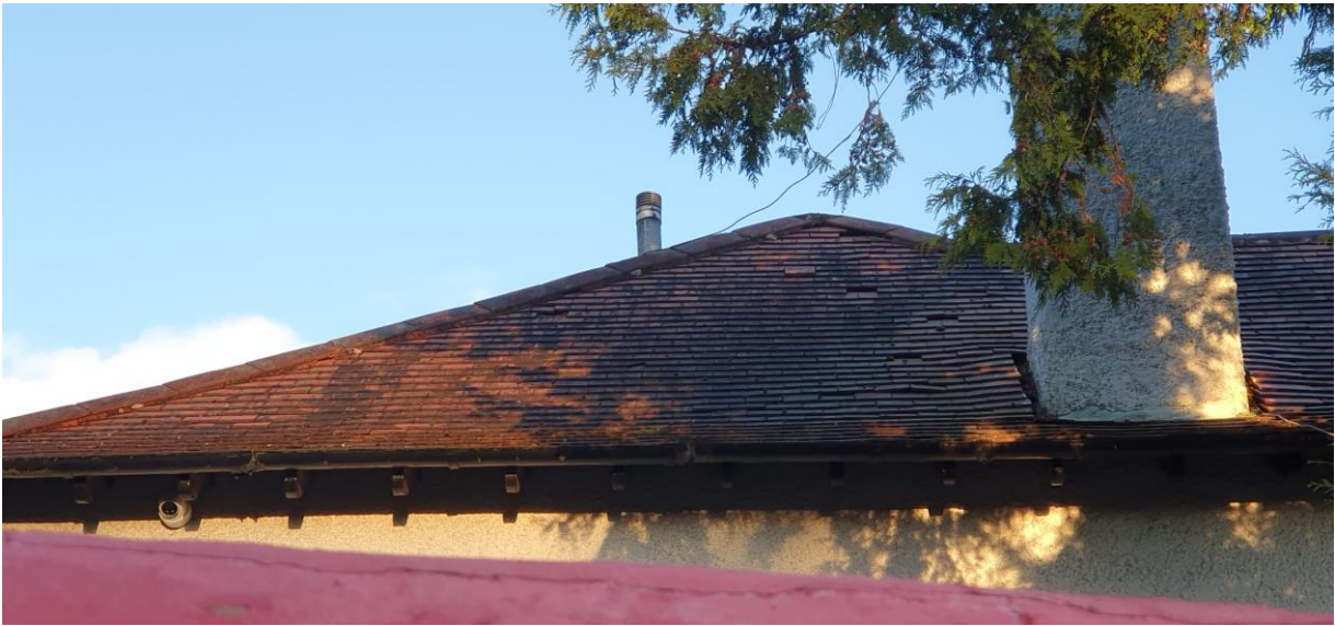
Plate 3. PRF – gaps where slates lost and under ridges on southwest gable
