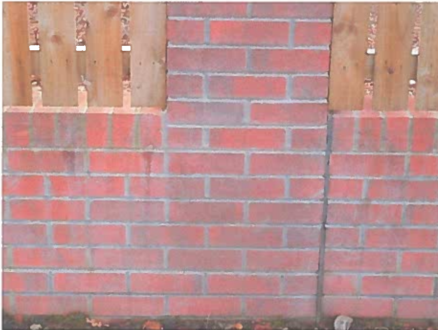
Typical Movement Joint. Slight Opening of Joint with Loose Sealant Evident
