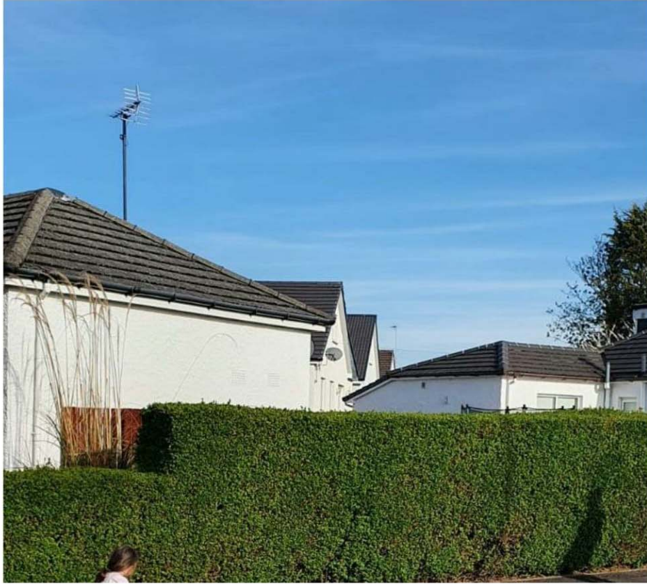
View of gable end at 27 and 25 Lawrence Avenue from west of 29 Lawrence Avenue
