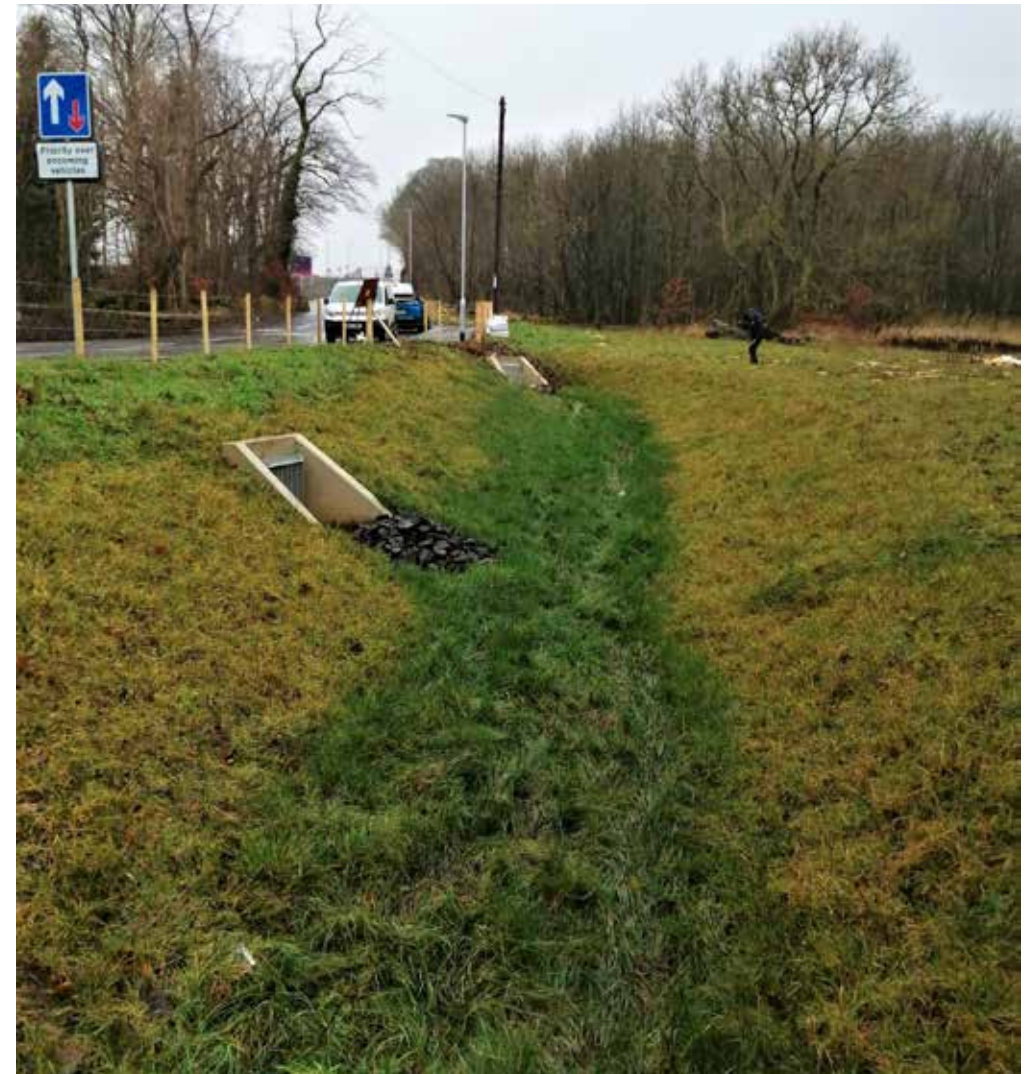
New swale constructed at Barrhead south. This simple piece of green infrastructure was cheaper to install than conventional underground piping. The grassy vegetation filters out silt and pollutants before water trickles into a nearby water course. The swale takes water from the near-by road and is maintained by the Road Service.
